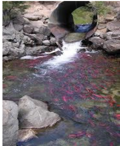
Figure 1. A poorly fit culvert blocking the migration of Kokanee salmon 10
