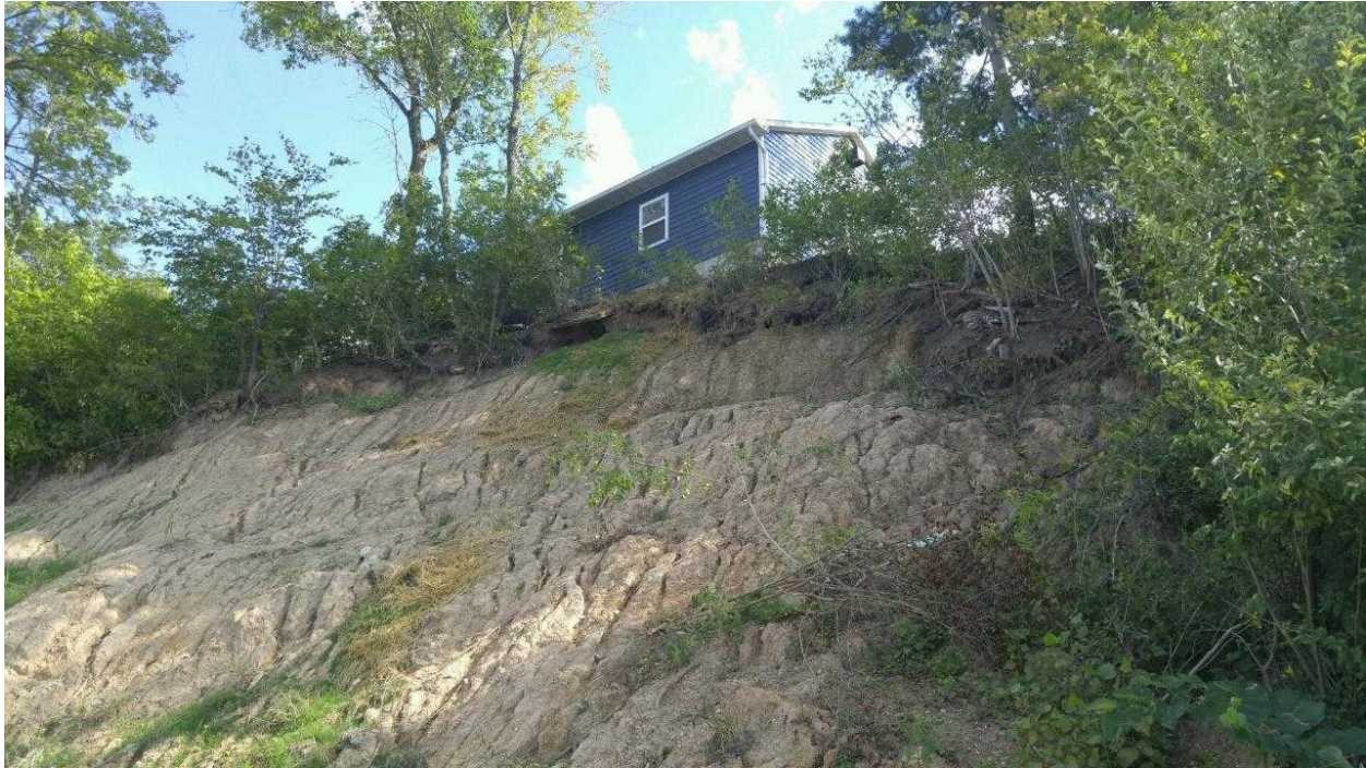
Figure 4. Slope erosion undercutting privately owned garage at Lake Charleston.
