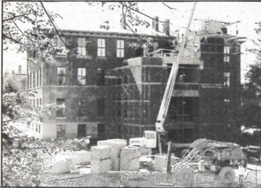
Engel Hall nears completion as the final touches go on the brand new elevator facility. Work on Engle Hall will be finished by the end of October. Across the campus, other construction projects are also in progress. (Photo by Dan Steger)
