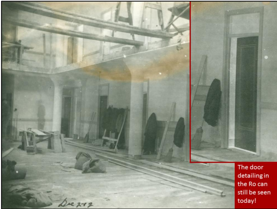
The Rotunda (Teresa Hall's 3 rd and 4 th floors) under construction. The door highlighted is currently the office of Parker Wheatley, chair of the Economics department, Main 335.
