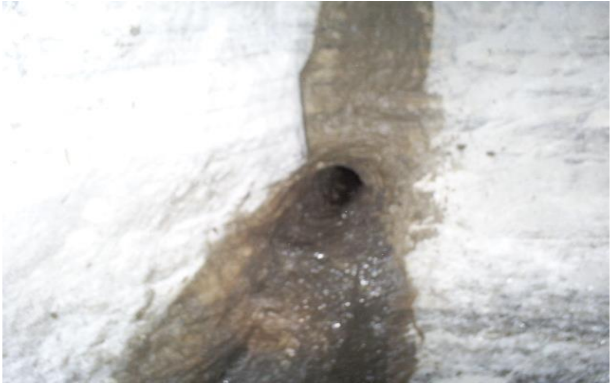
Figure 2. Water flowing from one of the three “boot holes”.
