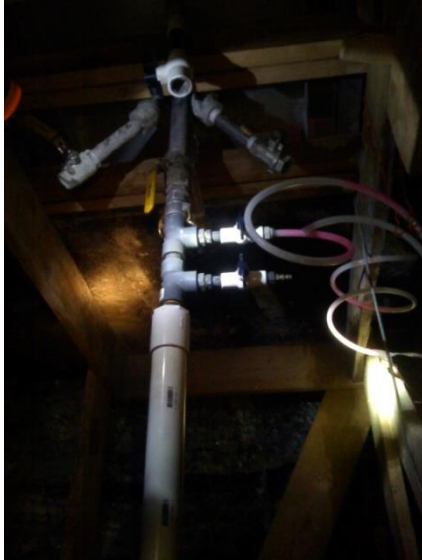
Figure 12. Air manifold for the pressure/volume test.
