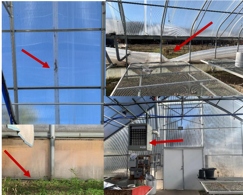
Figure 8: These images are all of the grounds greenhouse prior to the renovations. On the left are images of the paneling that show damaged seals and discoloration. The top right shows the collapsed wall of deflated air bags. And the last image shows the temperature control system which is not central to the space.
