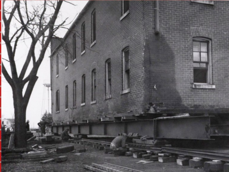
After moving, I served as a residence for men working for the monastery and college.
