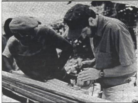
Teams from Global Volunteers work on building projects along with local residents in poverty-stricken counties in Mississippi. The program also offers two- and three-week volunteer opportunities in other countries. (Photo courtesy of CRT)
